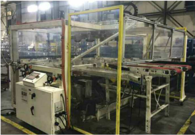
Overall view of the entry conveyors.
